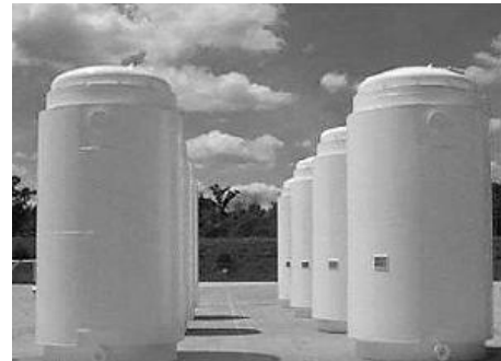
Above-ground fuel storage containers
